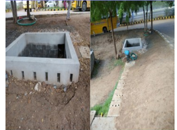
Figure 2. Rain water harvesting pit in college ground
