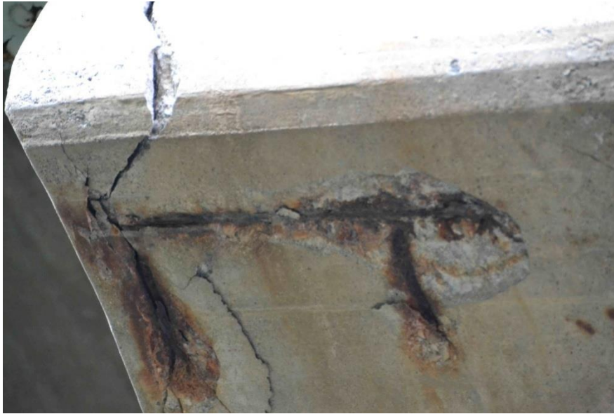
Fig.1.0 Corroded steel reinforcement possibly due to insufficient concrete cover
