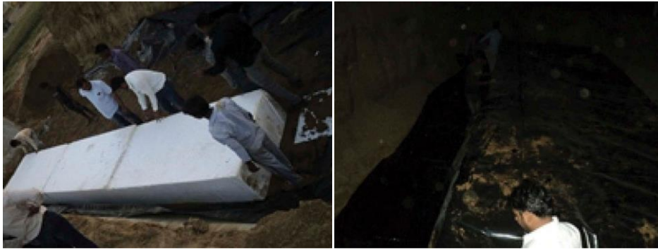
(c) Laying of Geo-foam block over geomembrane (d) Wrapping of geo-membrane over geo- foam for protection Against water and termilites
