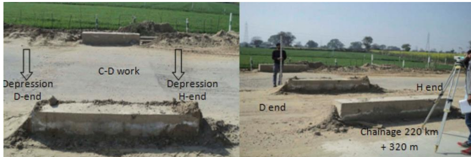
Figure 2 shows the settling and distress in the C-D culvert approaches.
