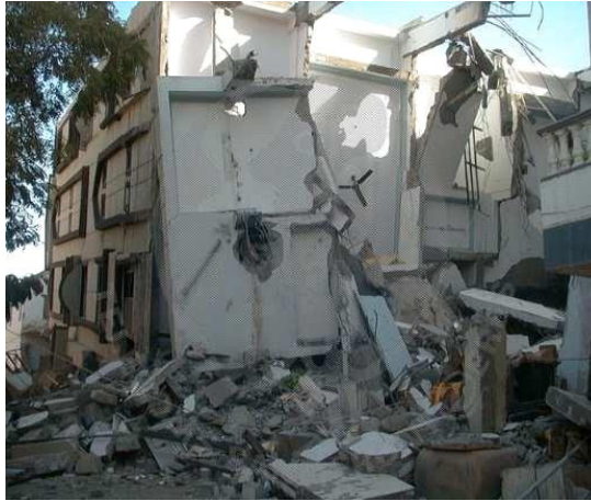
FIG.2BHUJ EARTH QUAKE IN INDIA
